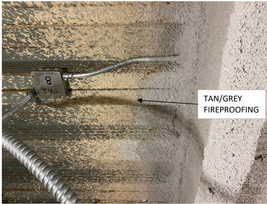
Photo 3: Two layers of spray-applied fireproofing was observed. These materials were not found to be asbestos-containing
