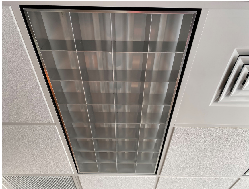
Photo 5: Typical lighting was LED or T-8 fluorescent bulbs with newer non-pcb electronic ballasts.
